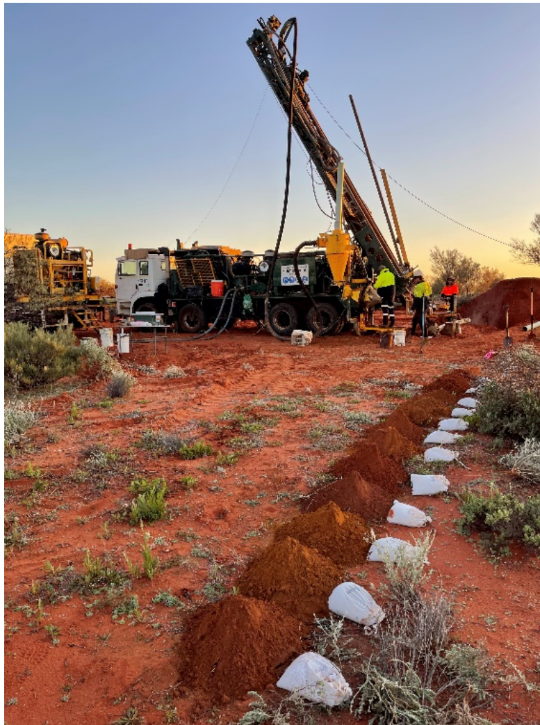
NDRC Drill Rig on Site at Solis Prospect, Island Gold Project (July 2022)
