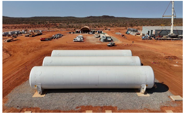
Figure 16: LNG storage vessels
