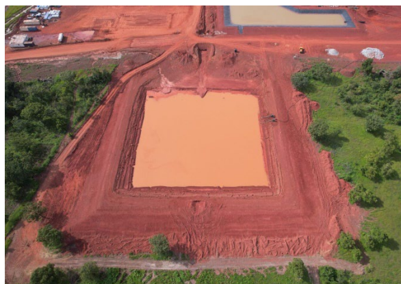
Image 7 - Plant drainage and sediment pond
