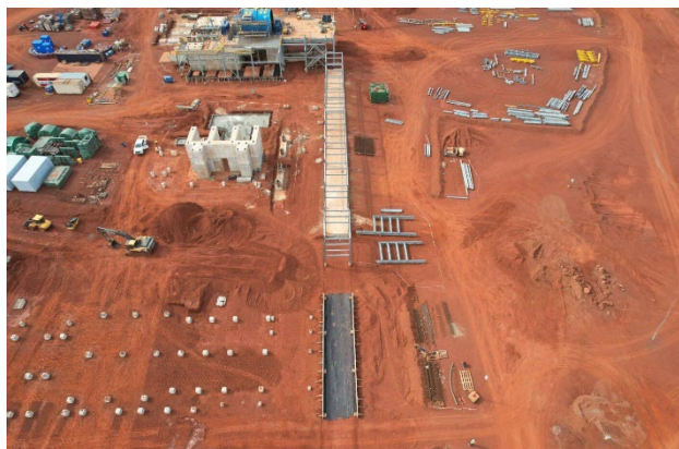
Image 8 - Wet plant and pipe rack
