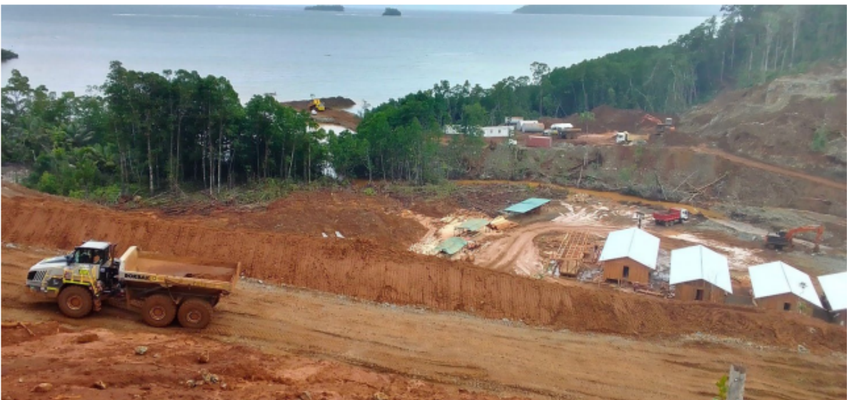
Mining truck and camp in foreground, mining contractor site in the middle-ground and wharf construction in the distance.
