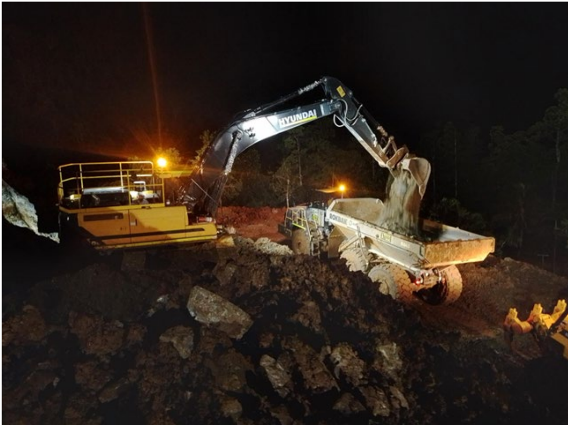
Two-shift (24-hour) operations commenced utilising lighting plants in line with the long-term operational requirement for continuous operations
