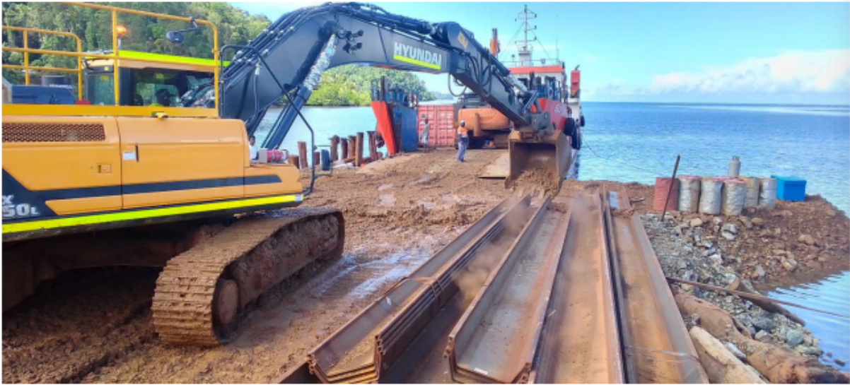
Sheet piles to be used in construction of the Wharf arriving at Kolosori
