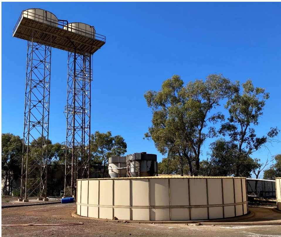
Figure 37: Water Infrastructure on Site
