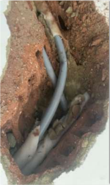
Kinked or damaged pipes, pipes overlapping; tight bend on back pipe
