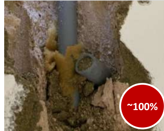
Lagging not impermeable (and at times non-existent)
