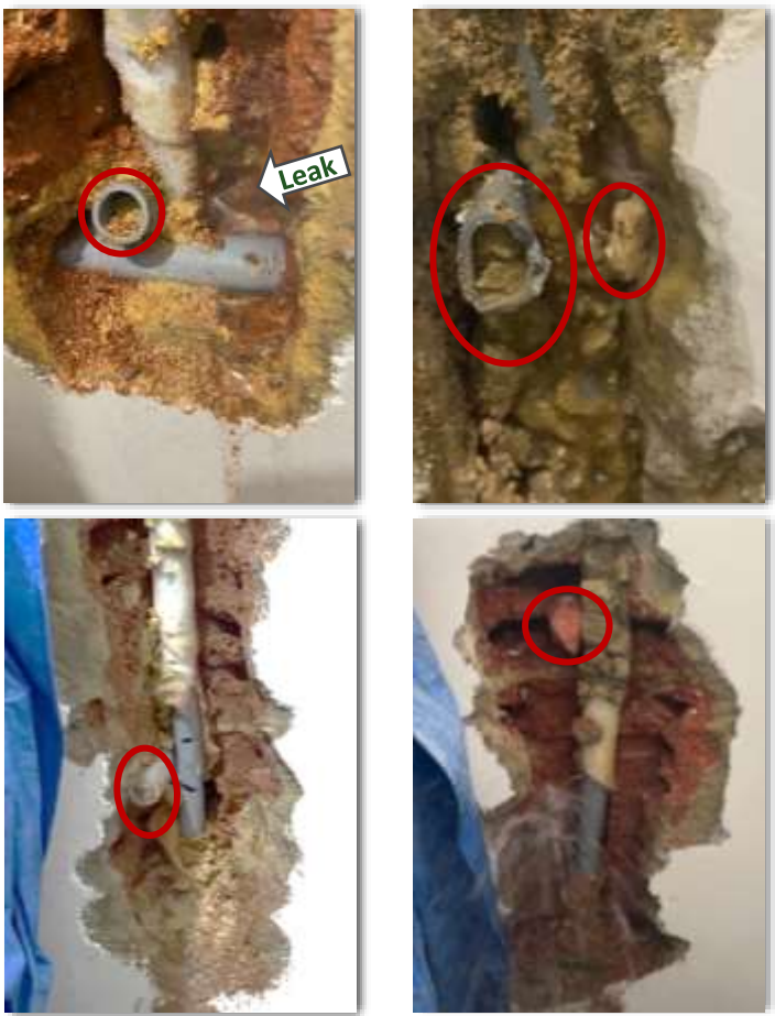
Inadequate movement and damage to pipe caused by pegging left in chase
