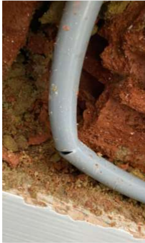
Kinking or damaged pipe not replaced per guidelines
