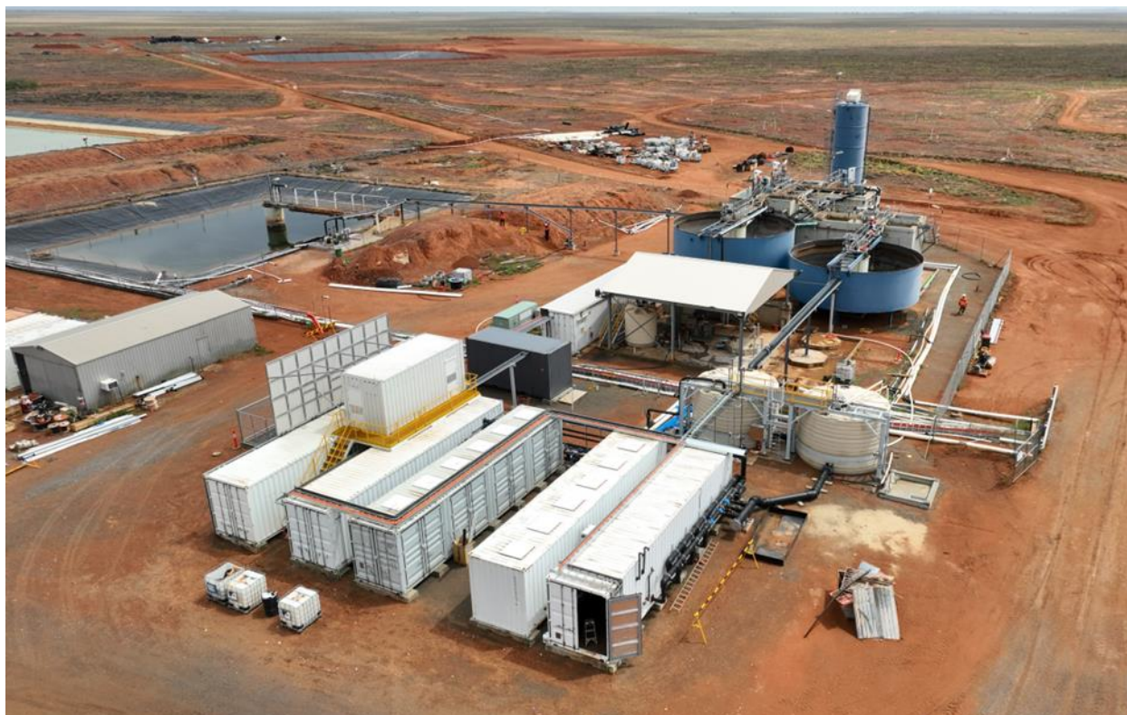
Image 2: 250m 3 /hour RO Plant and Water Treatment Plant
