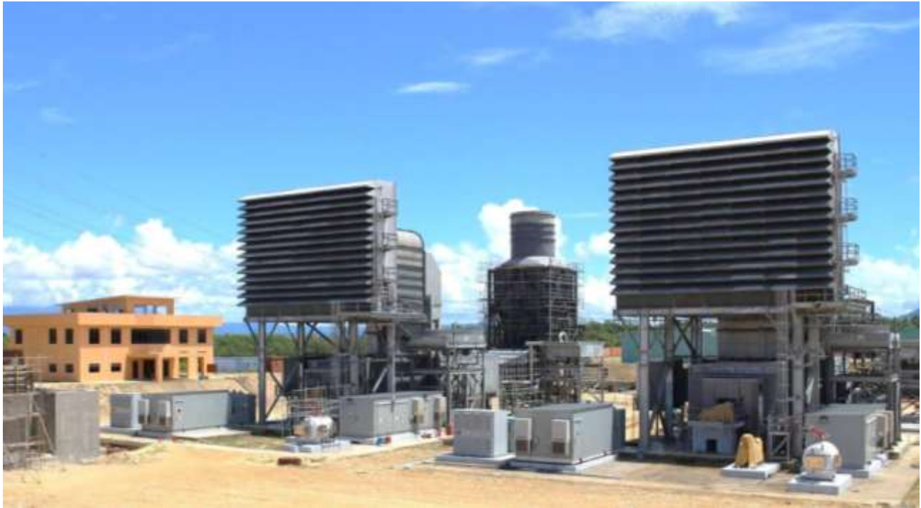
Philippines Power Plant 2 x 200MW
