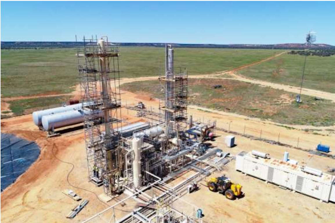
Eromanga Gas Plant
