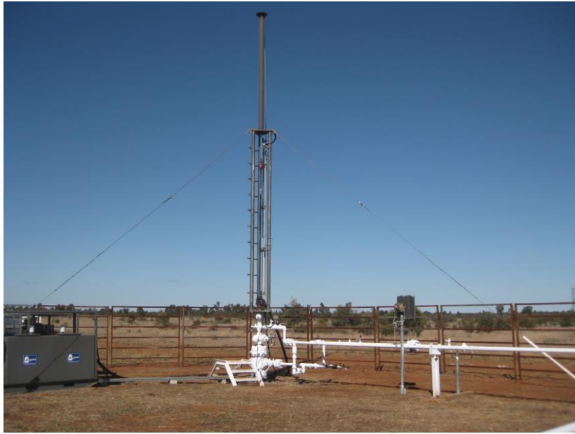
Figures 6 – New Royal 8 Rod Pump facilities installed June 2023
