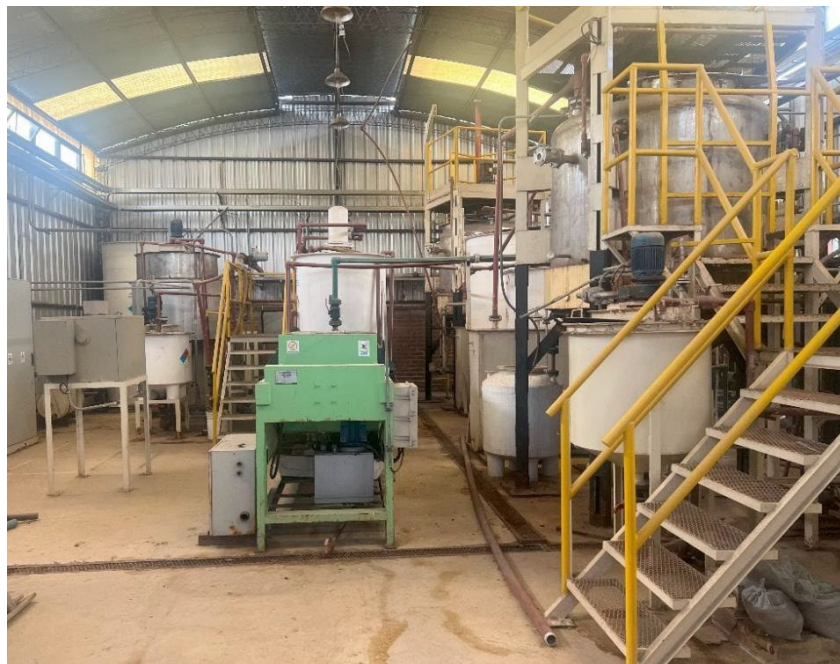
Figure 11: Pursuit's Pilot Plant during site visit March 2023
