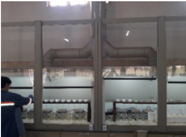
Fig 13 New exhaust system
