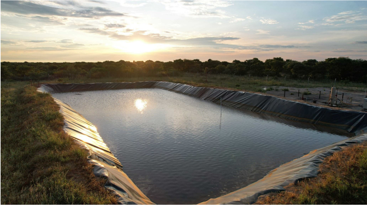
Figure 7 - Serowe 3 Flow testing evaporation pond.
