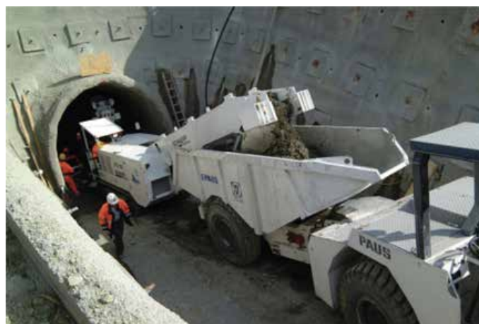
Figure 7: ITC loader paired Paus bi-directional haul trucks to be used in the trial mining
