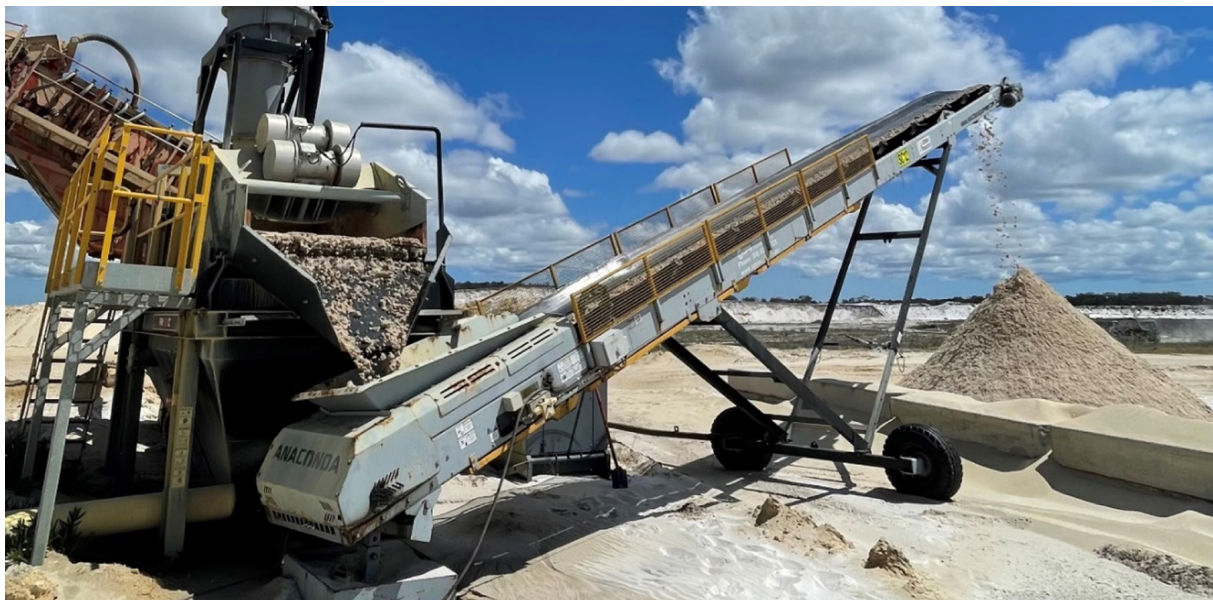
Figure 5: Third party Sand Wash Plant processing 20-tonne bulk sample from Stockyard Silica Sand Project
