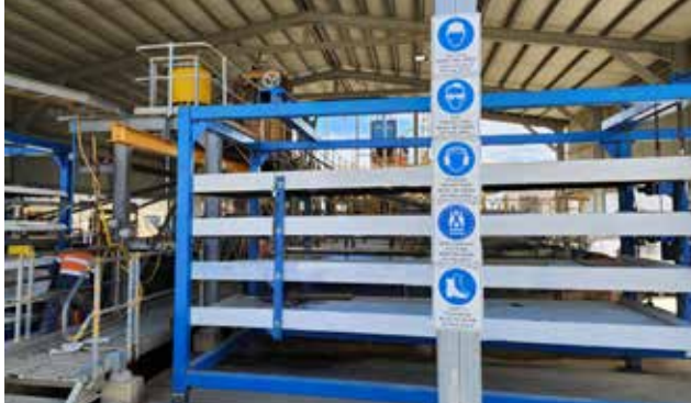
Eight additional shaker tables have been installed and commissioned to increase processing capacity.
