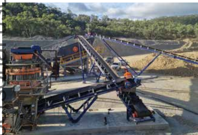
Crushing and Screening Plant with the Cone Crusher at the forefront.
