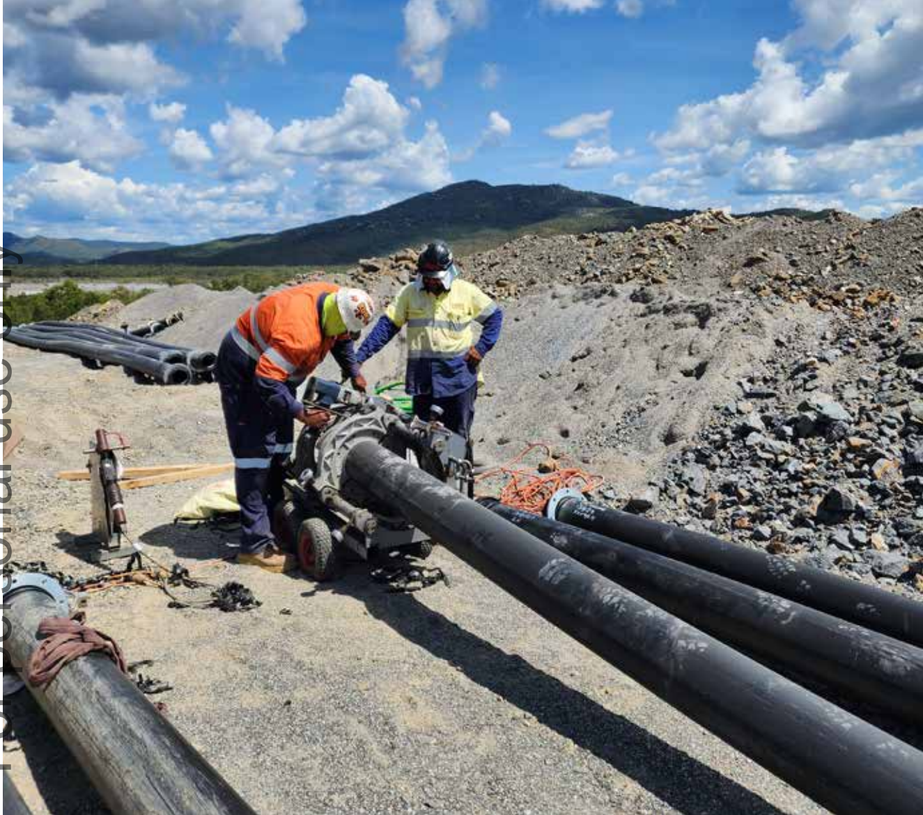
Efficient transportation of fines from the crushing Plant to the Gravity Plant has been achieved through the successful implementation of slurry lines.
