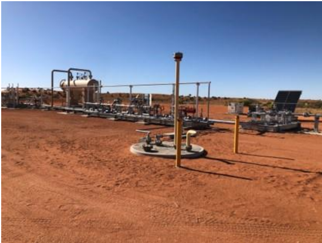
Vali field separation and metering facility
