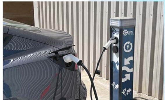
EV Charger at Sims Metal Kwinana
