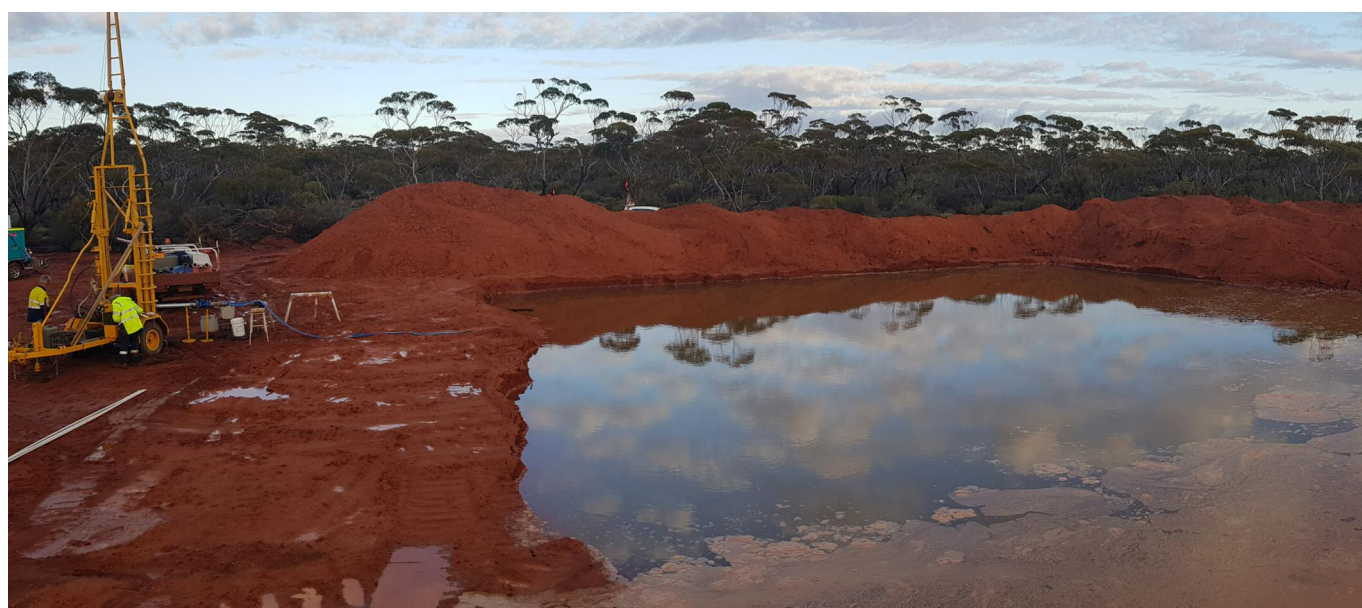
Photo above: Large water sump from Goongarrie Hub production bore drilled in July 2022.
