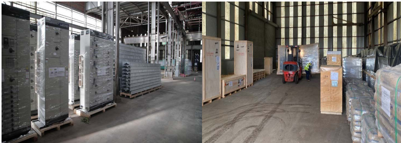
Process Control Software (PCS) Panel Delivery
