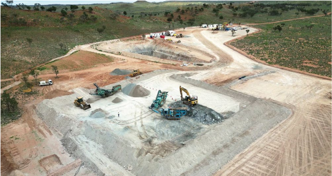
Figure 3 – Multi-stage crushing plant processing ore stockpile in preparation for milling
