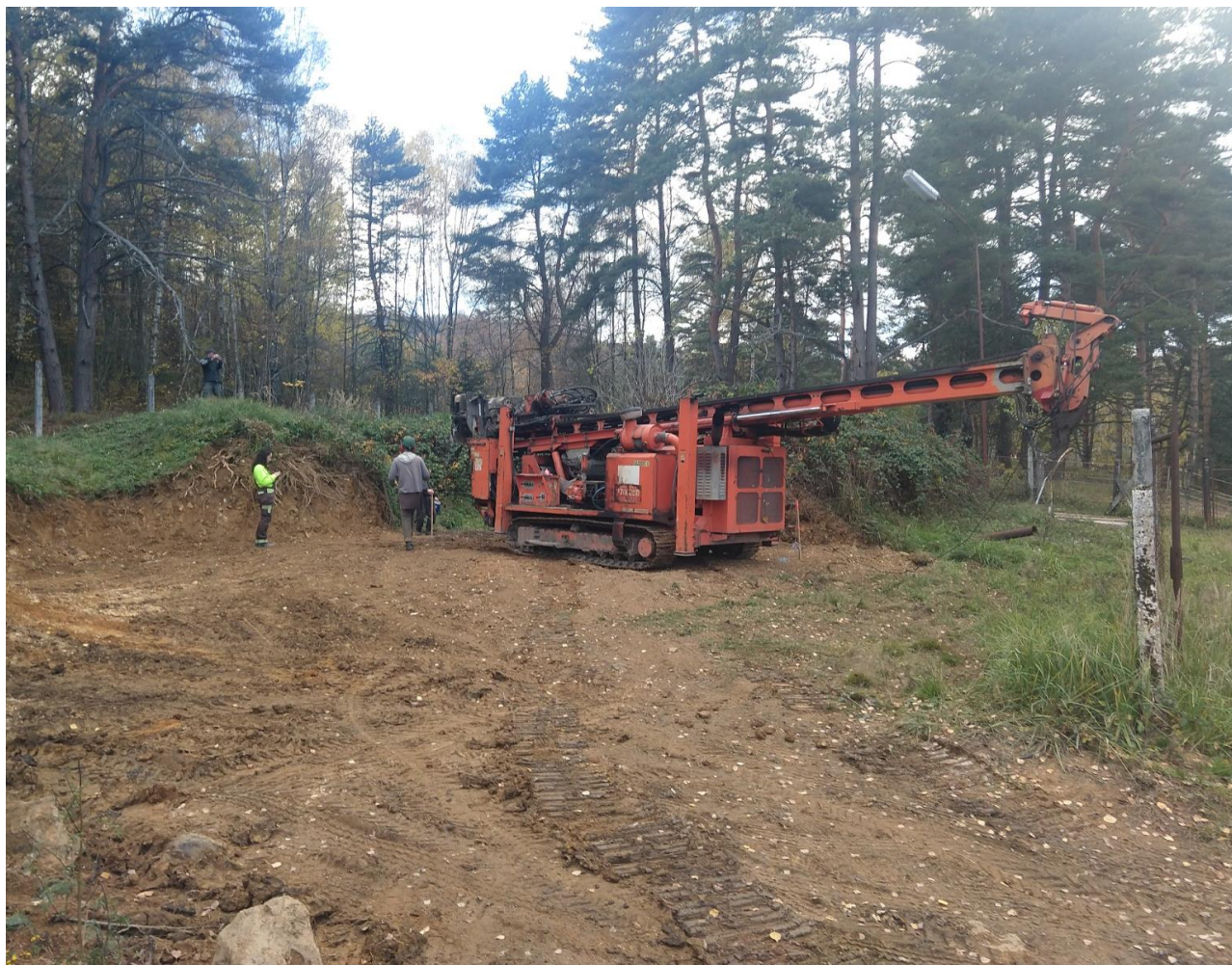
Figure 16: Diamond drill rig set up at the first target area, site preparation completed, location of drill hole SSD-01
