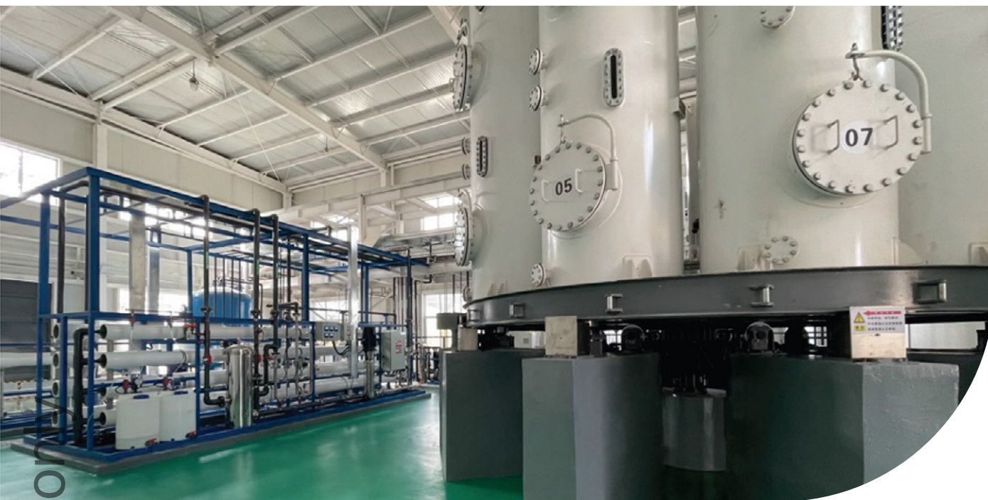
Figure 3: Lanshen DLE test facility in Xian, China
