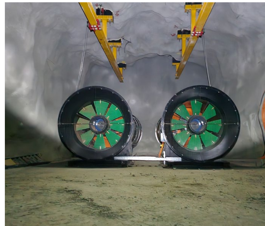
Installed Booster Fans
