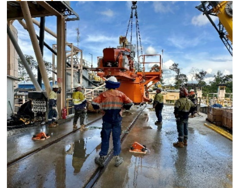
Figure 6 | Okvau Maintenance Personnel
