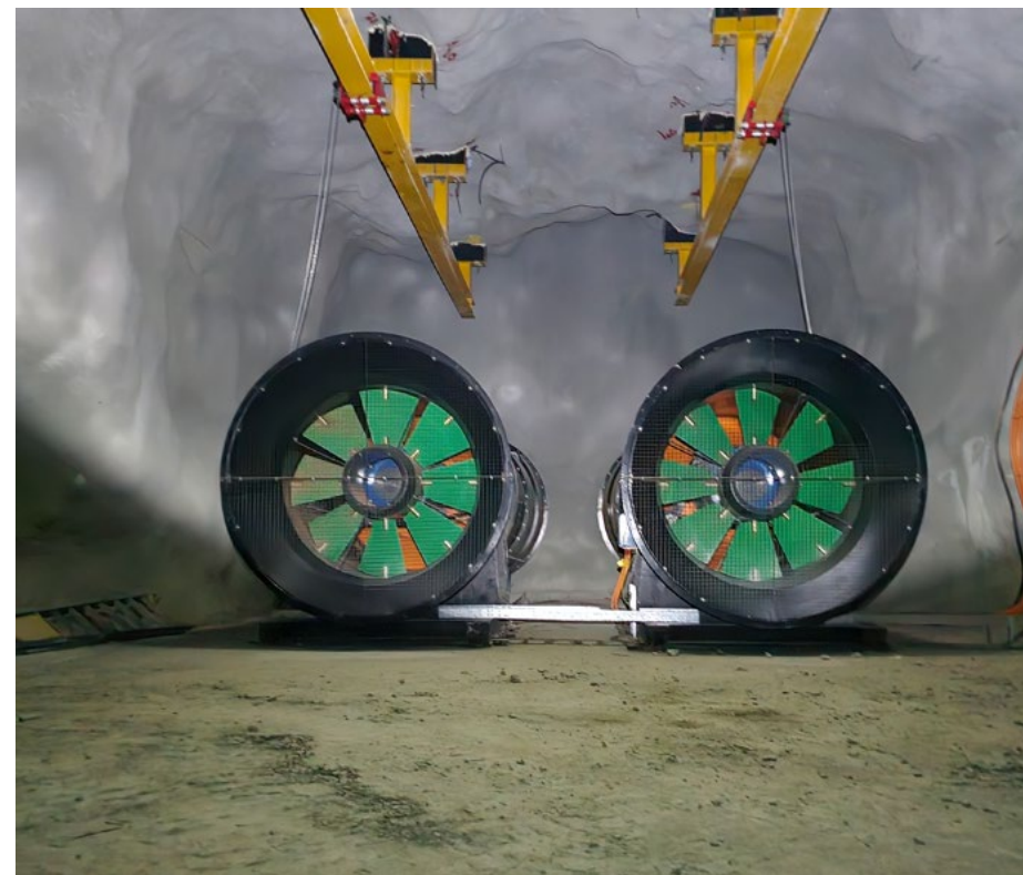
Installed Booster Fans
