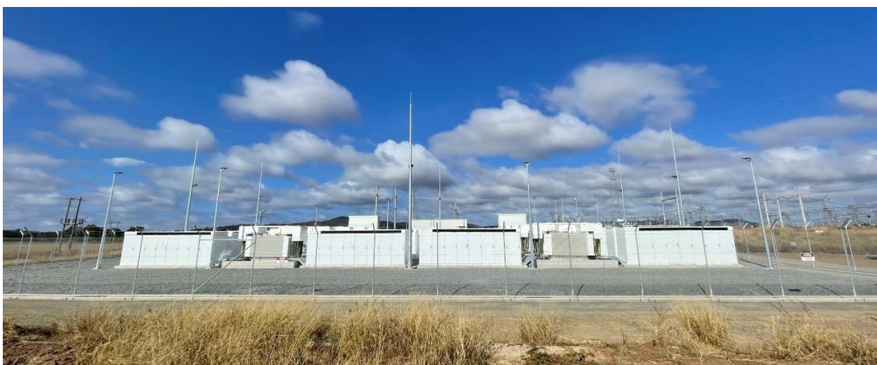
Figure 1: 50MW/100MWh Bouldercombe Battery Project
