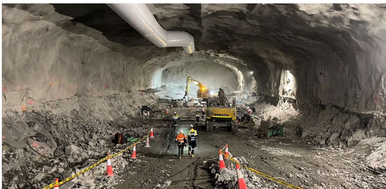
Figure 2: Power Station Cavern at the 250MW/2,000MWh Kidston Pumped Storage Hydro Project
