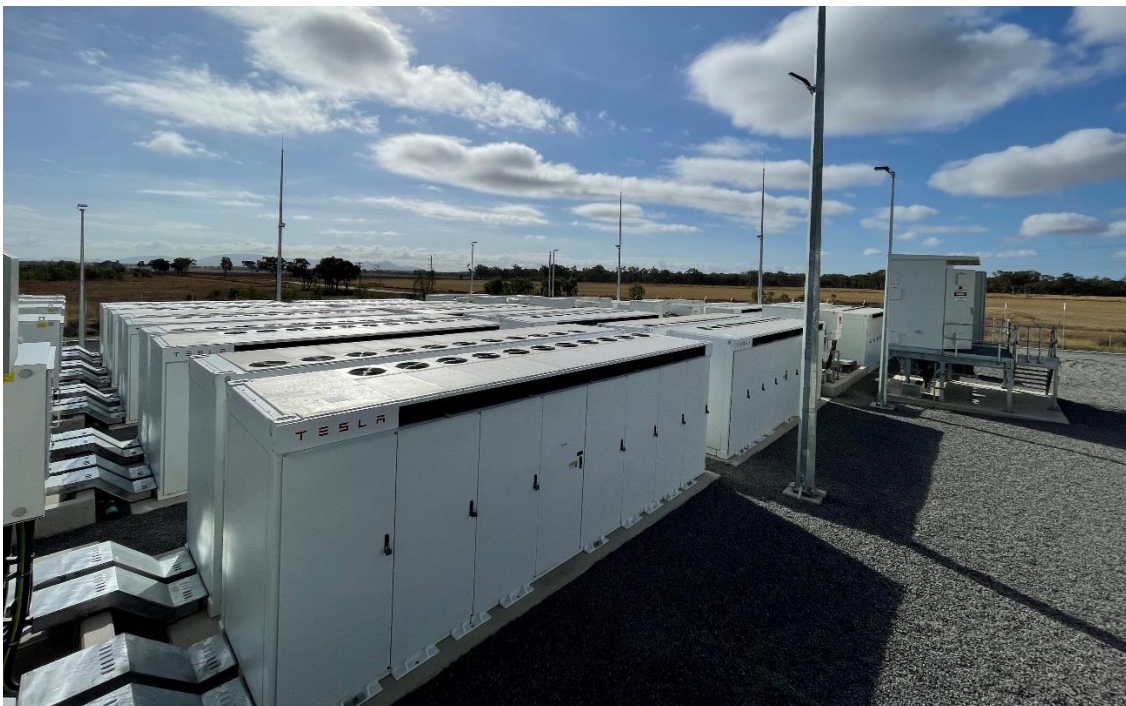
Above: 50MW/100MWh Bouldercombe Battery Project, Central Queensland
