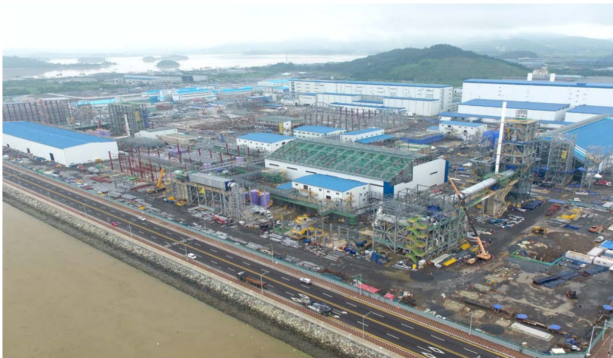
Image: Construction site at the Lithium Hydroxide Processing Facility in South Korea as at 20 July 2023
