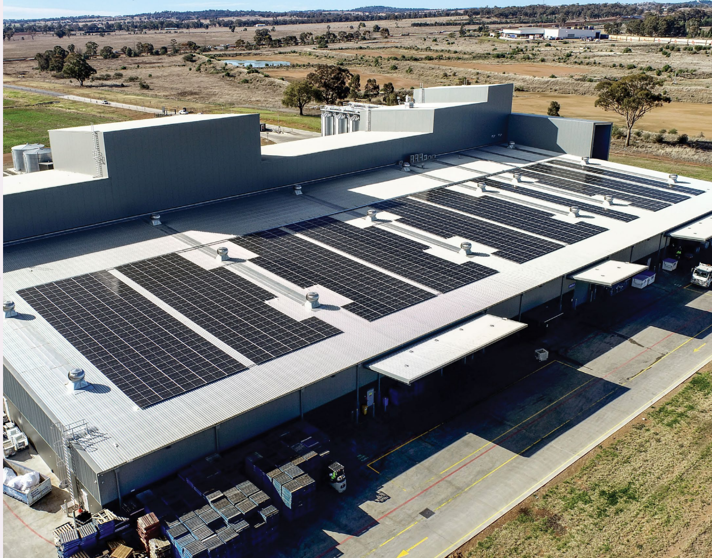
Roof-mounted solar array at Parkes, NSW
