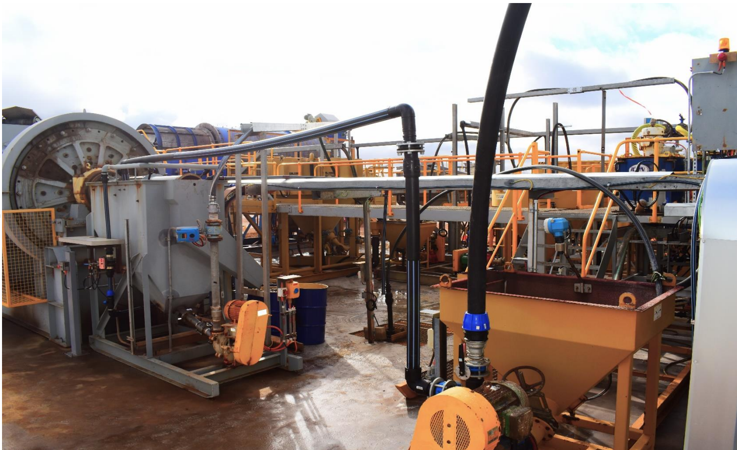
Figure 1: Classic Minerals Kat Gap processing plant commissioned.
