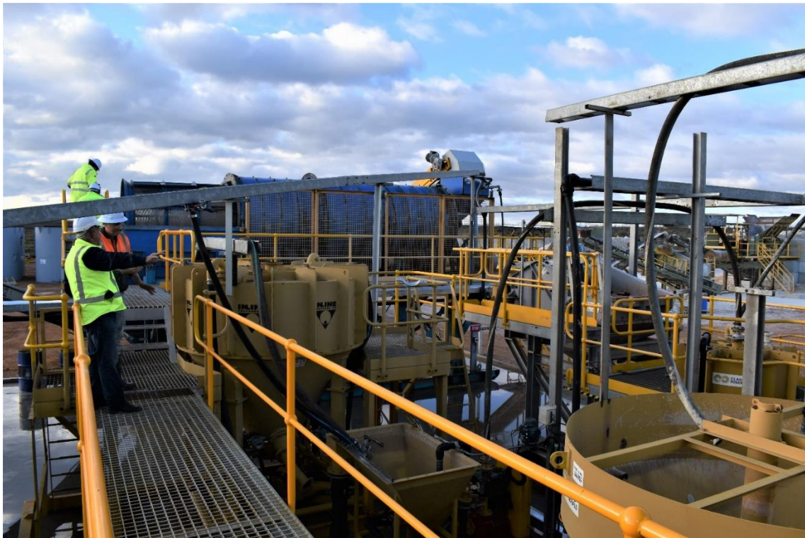
Figure 6: Classic Minerals Kat Gap processing plant commissioned.
