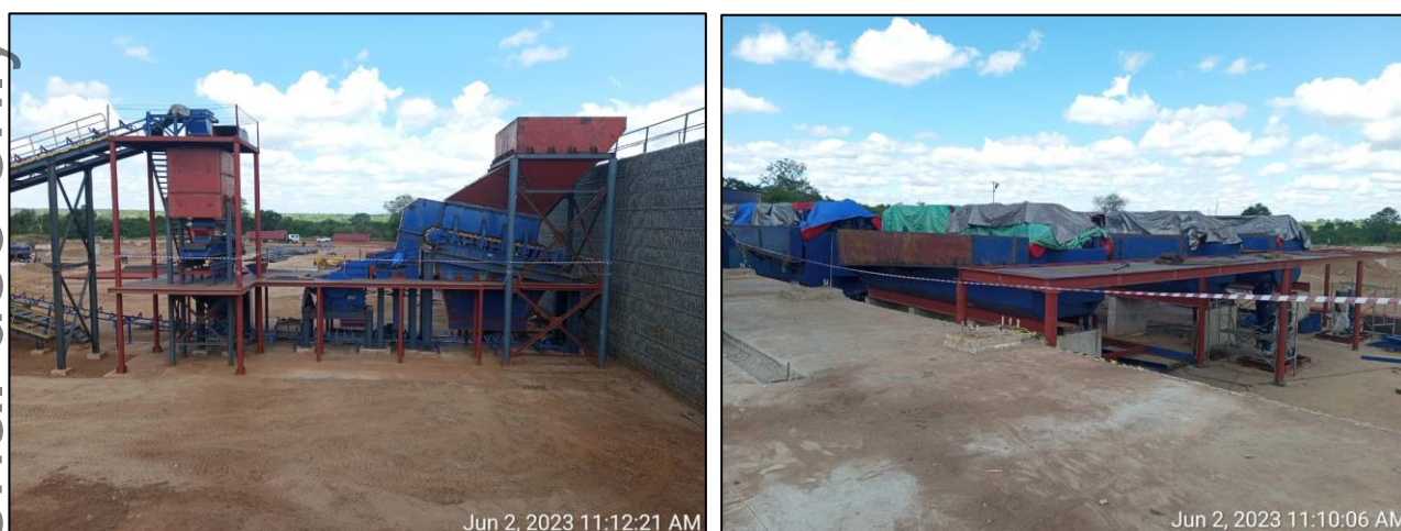
Figure 2: Mechanical completed crushing circuit (left) and the platforms around the flotation circuit (right).
