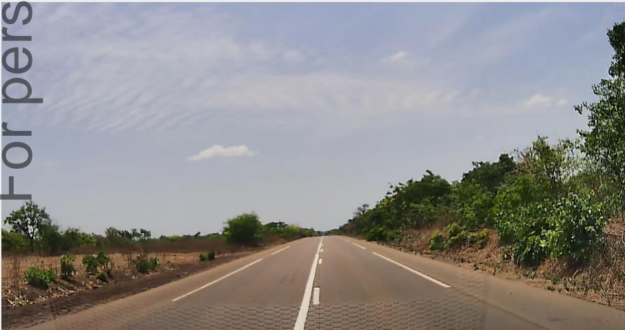
Typical road condition - Tingrela area
