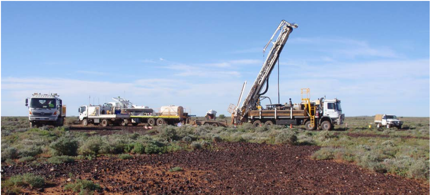
Figure 4 Drilling copper anomalous gossan outcrop (dark brown ironstone scattered in the foreground) at the Johnson Dam prospect lying 14 km south-southwest of the Kalkaroo copper-gold-cobalt deposit.
