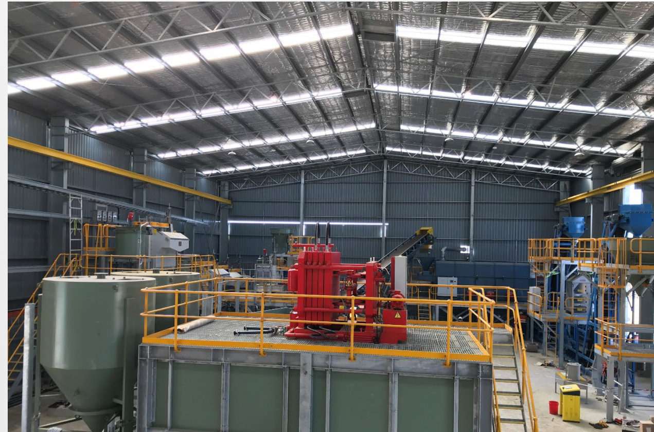
Concentrate dressing, drying and bagging area
