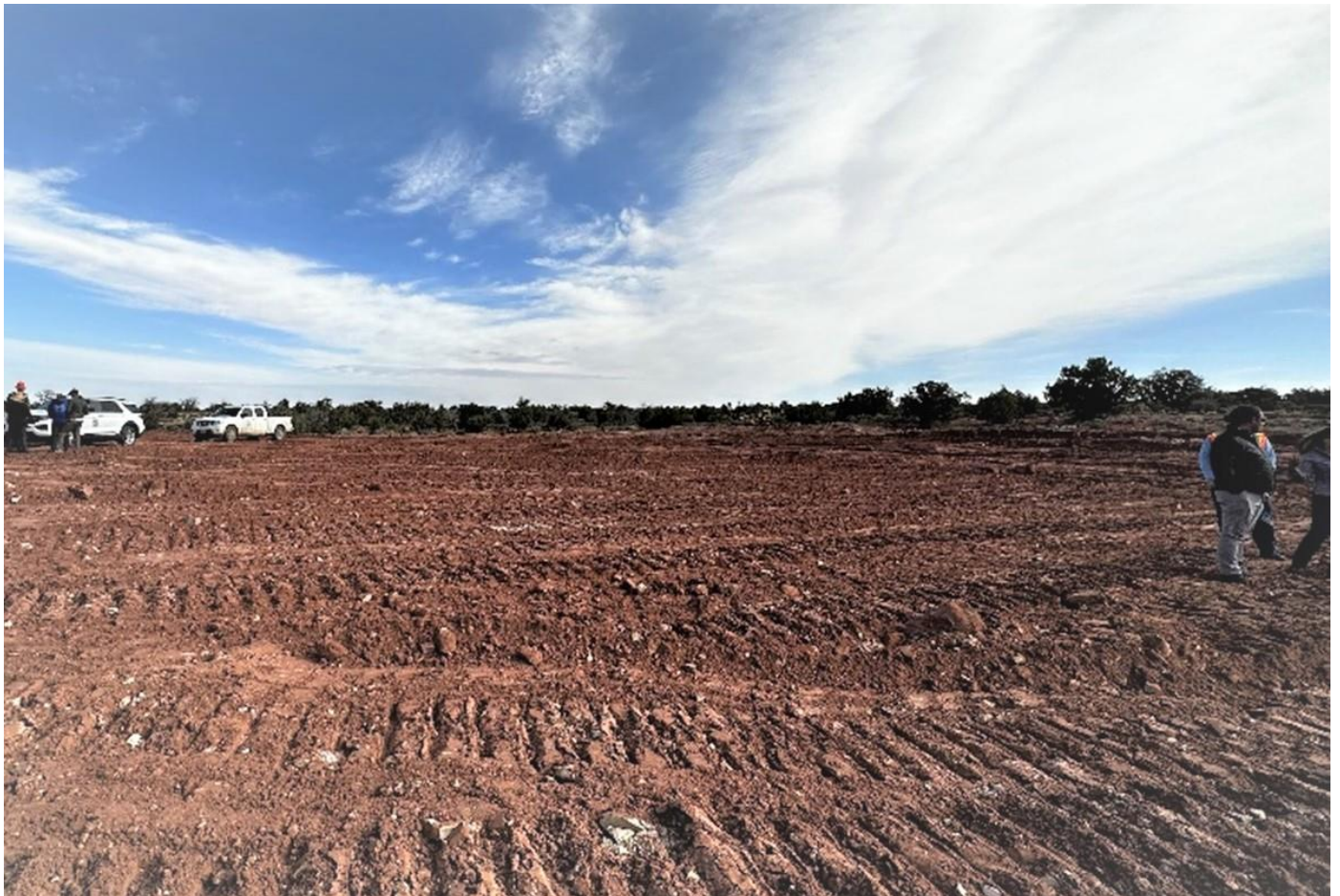
Figure 1: Federal and State personnel inspect the re-instatement works on the Mineral Canyon pad.
