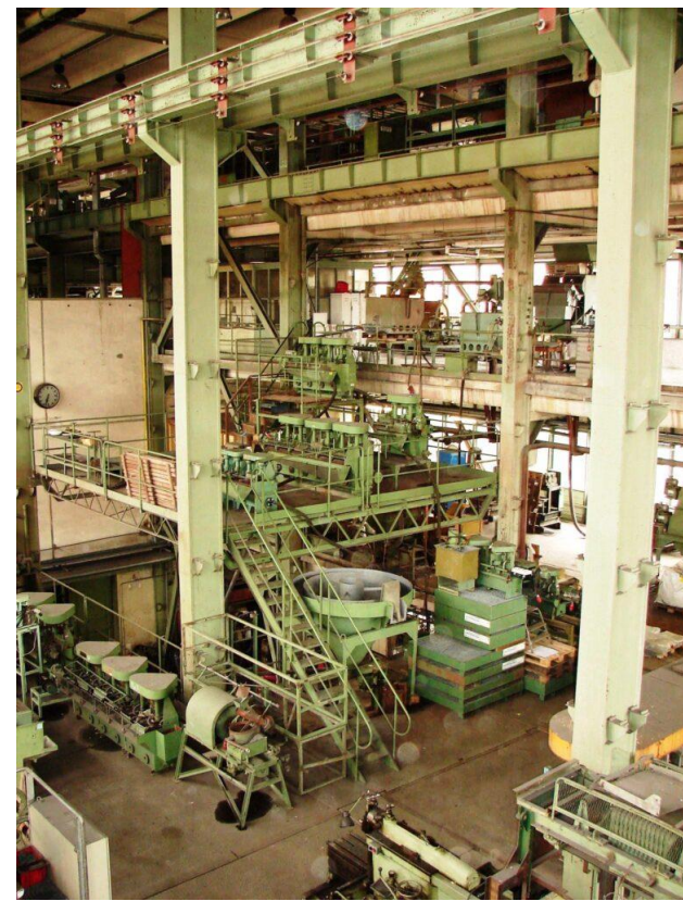
Bulk flotation facility Germany
