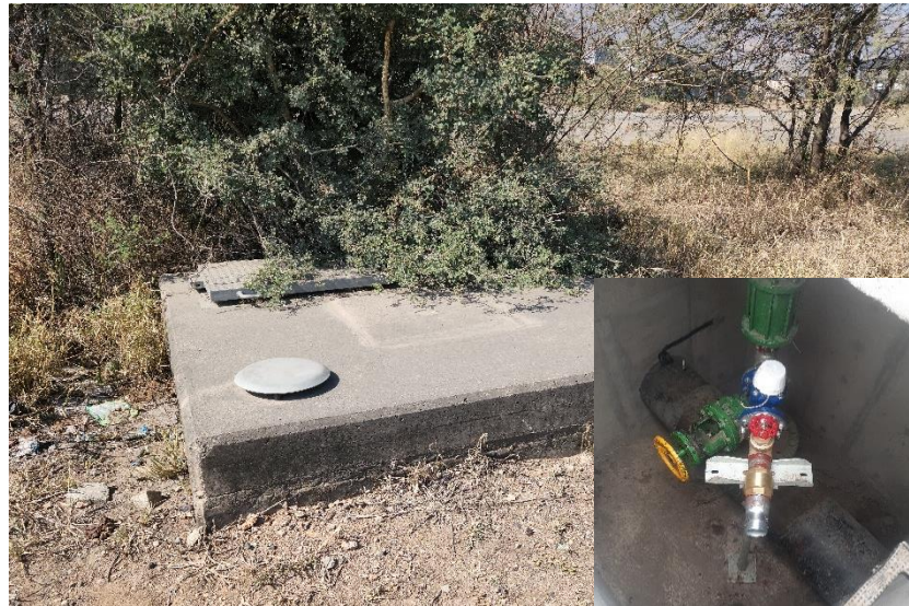
Water Source at Entrance
