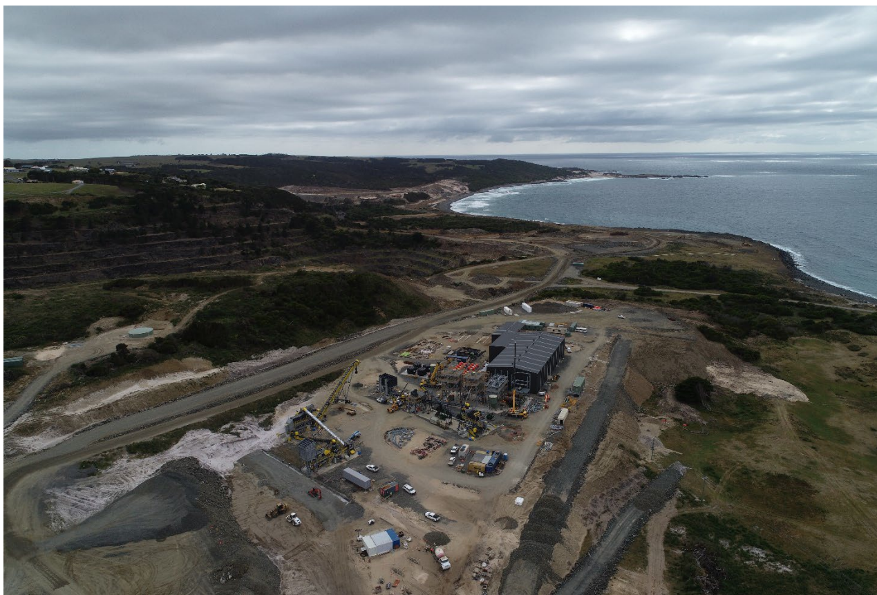
Figure 1 - DTM Process Plant December 2022 (looking North East)
