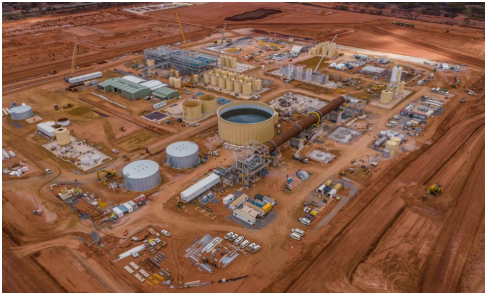
Feed Hood lower platform completed for bricking, Soda ash silo complete and installed, MgO outer concrete tank walls completed, MgO silo structures in place, Carbonation civils completed and tank installation commenced, milk of lime tank installed.
