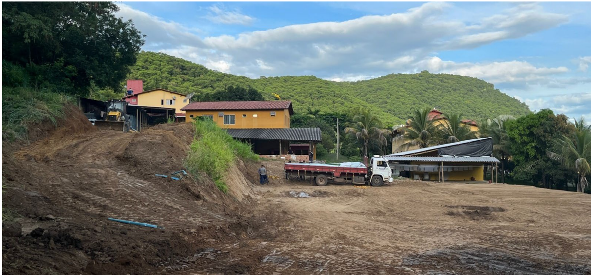
Figure 5: Site construction work underway in early January 2023, to expand the existing core processing and storage facility on site at the Salinas Project in Brazil
