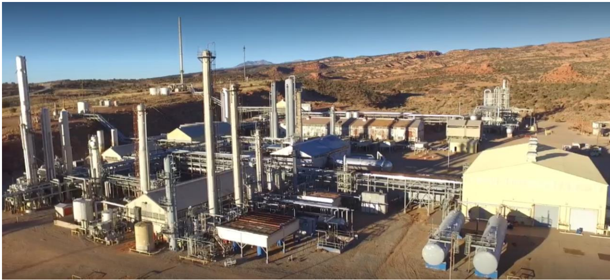
Figure 2: Paradox “5.5 Nines” Resources Lisbon Valley Gas Processing Plant.
