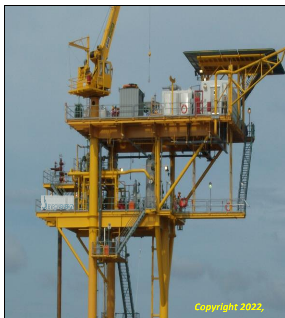
Recently purchased platform deck while still in service. US Gulf of Mexico
