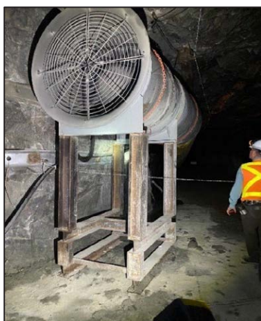
Underground secondary fan
