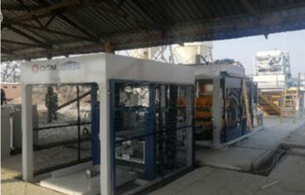
QT 6 multipurpose plant
