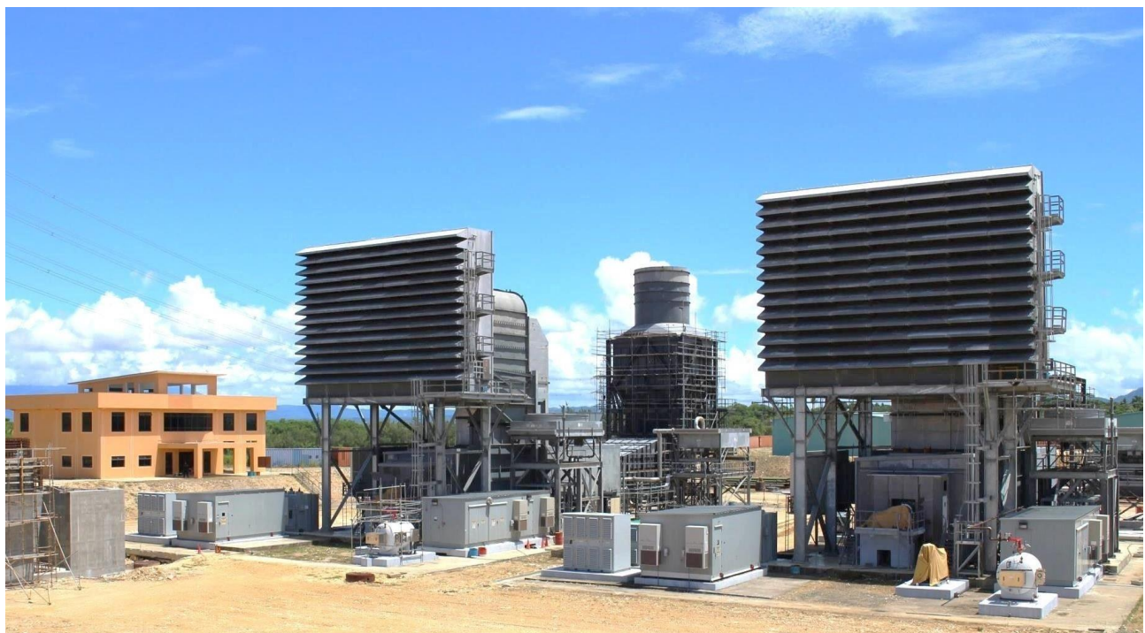
Philippines Power Plant 2 x 200MW
