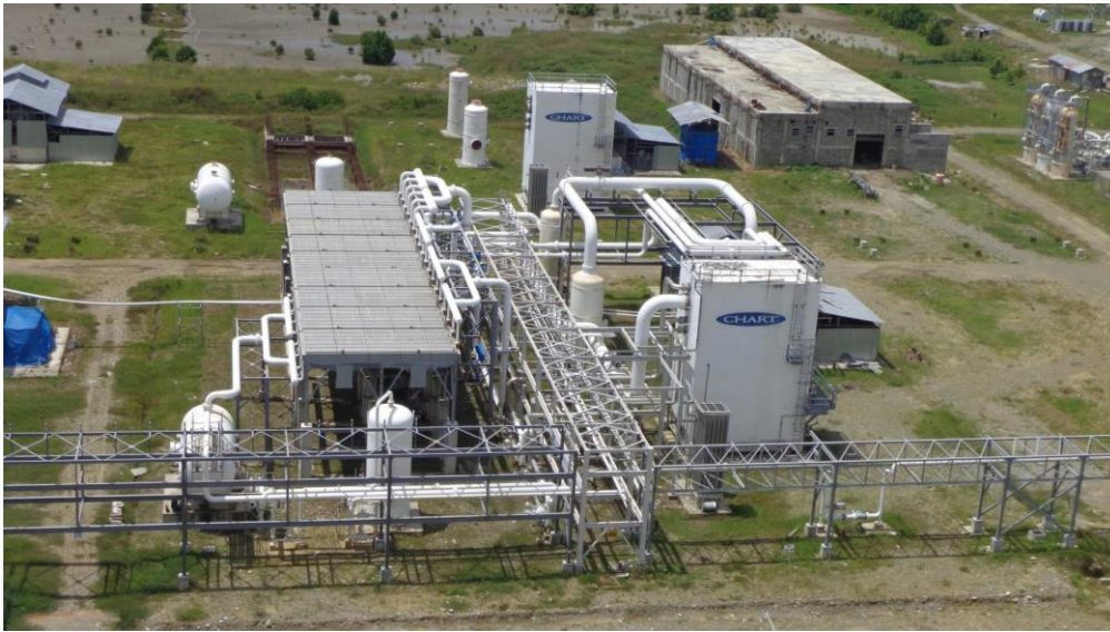
Main Processing Plant Area
