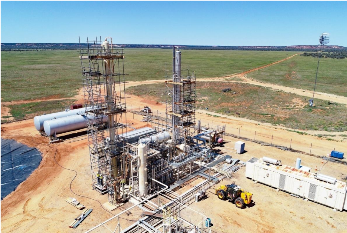
Eromanga Gas Plant
