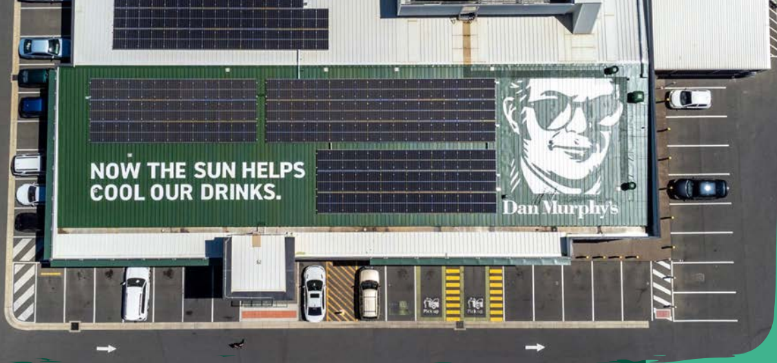
Following the Sun The roof of the prominent Brickworks Dan Murphy's, positioned directly under Adelaide Airport's flight path, celebrates the installation of its new solar panels.
