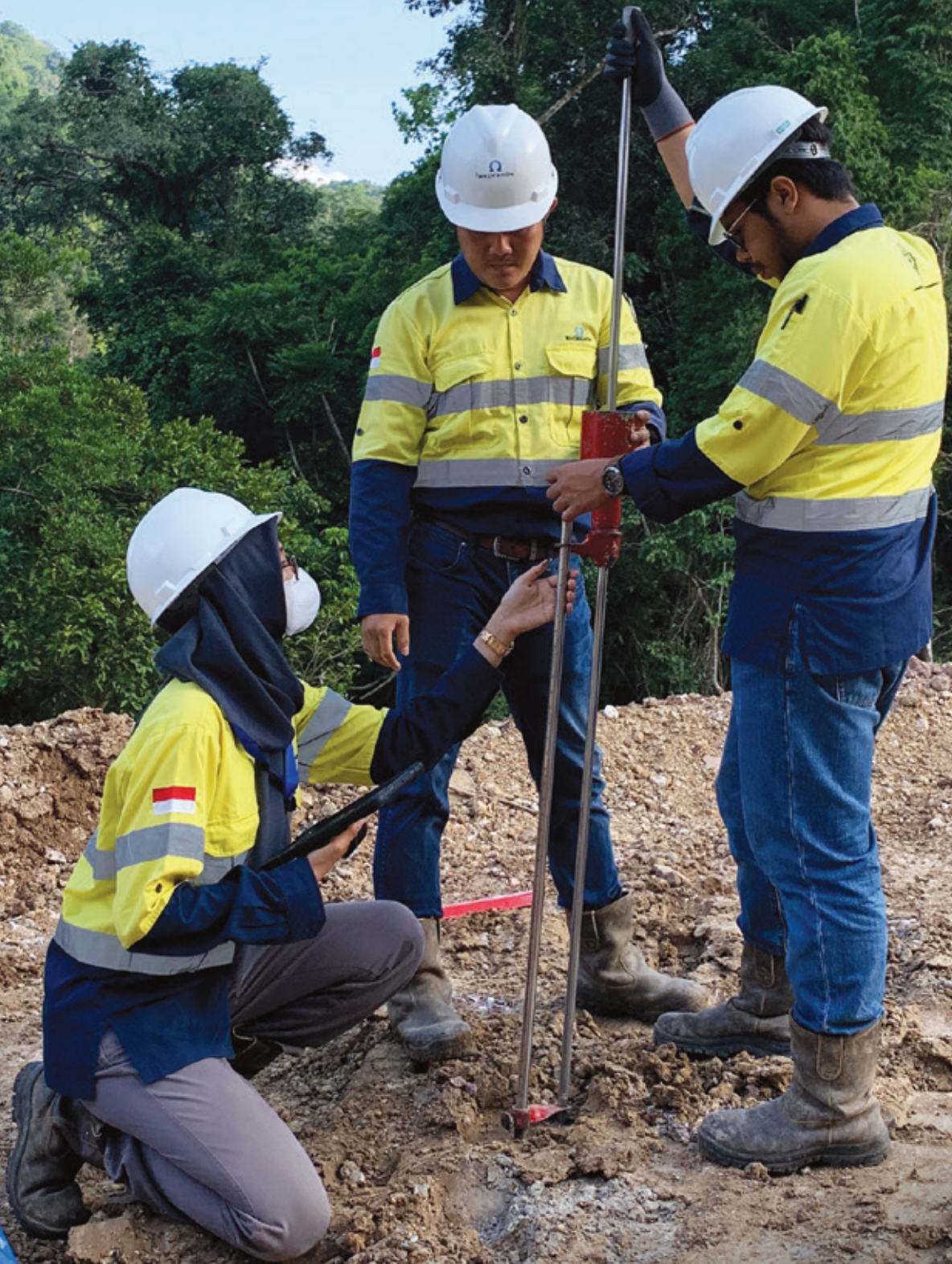
The Martabe Engineering Team checks the road quality during construction by reading the Dynamic Cone Penetrometer tool to estimate the load-bearing capacity.
