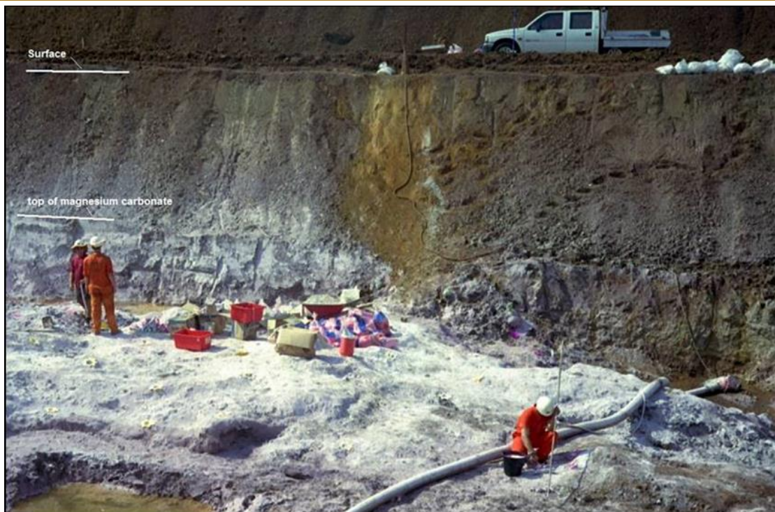
Figure 5 Test mining of magnesium at Winchester during the wet season (preparing to blast Level -1)
