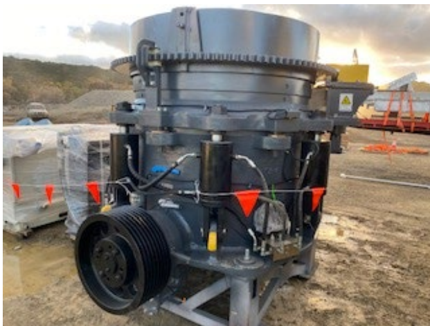
Figure 4 - Secondary Crusher on Site
