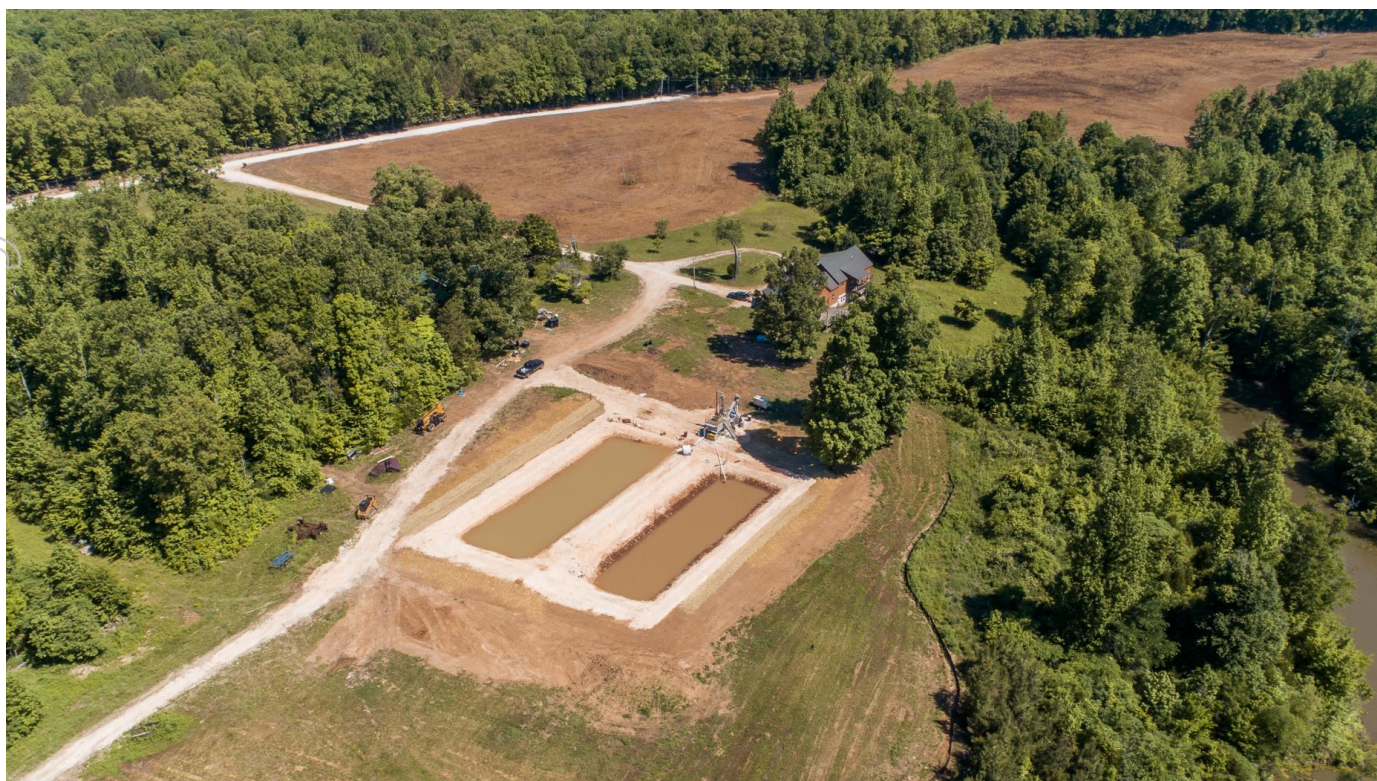
Figure 12: Titan Project Mineral Demonstration Facility.
